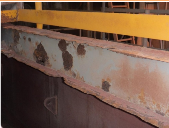
Loss of cross section to parts of structural steel beams
