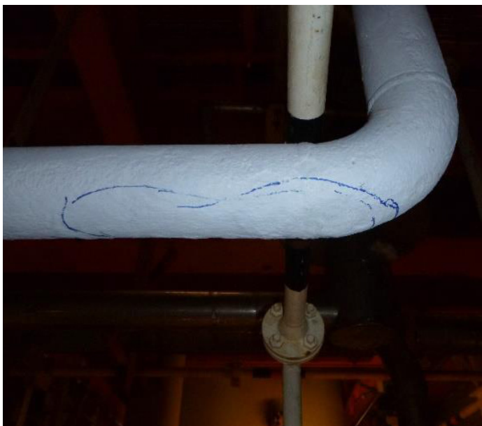
Reduced wall thickness was identified along a 560mm section of the line
