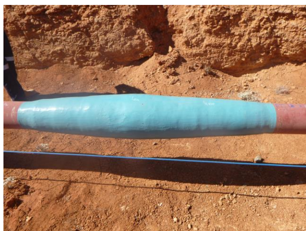
Previous composite repair - internal corrosion defects identified at either end of the repair.
