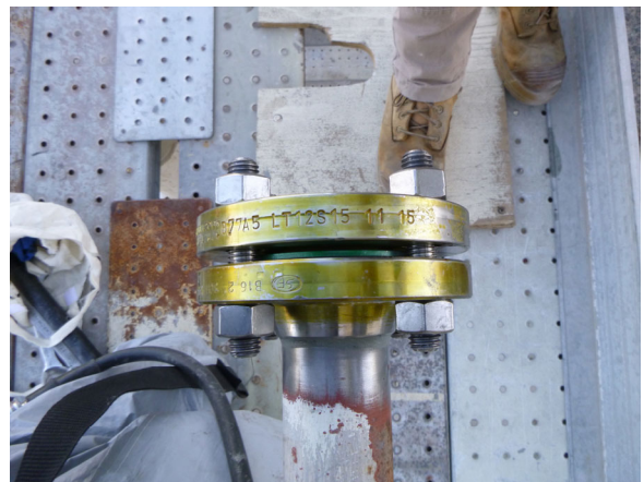
Completed installation including a blind flange
