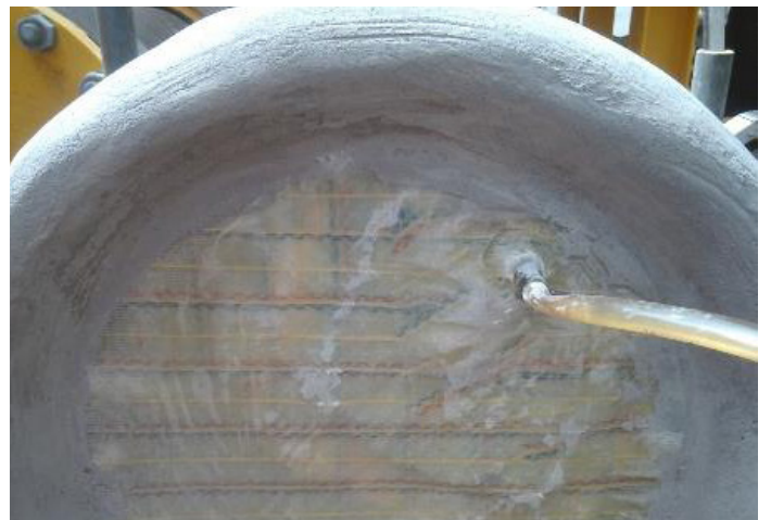
The engineered repairs were designed for a 19-year life, matching the lifetime of the original piping
