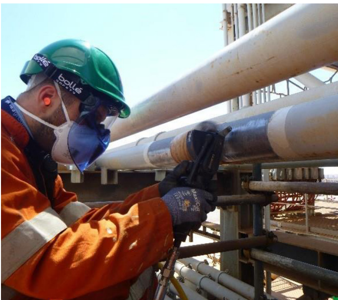
Temporary repair wraps were left in place, allowing the lines to remain active
