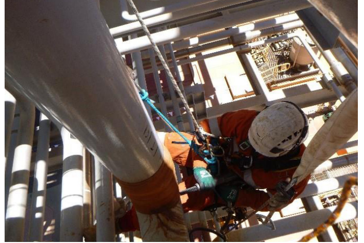
The repairs were completed on ropes by ICR IAS JV Application Specialists
